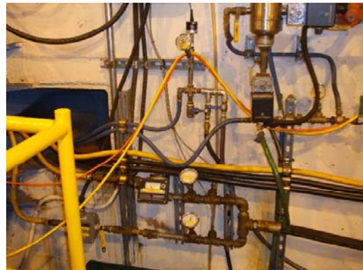
Photo 16: Air/water distribution headers
