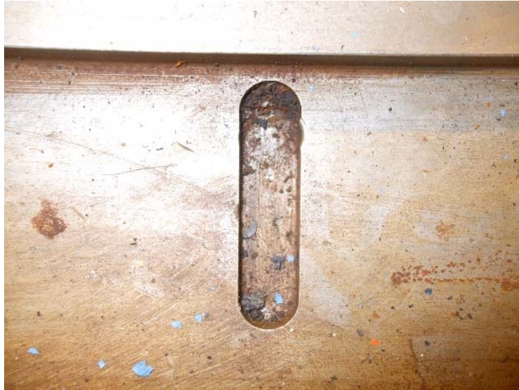
Photo 14: Damaged slot for anti-rotation pin
