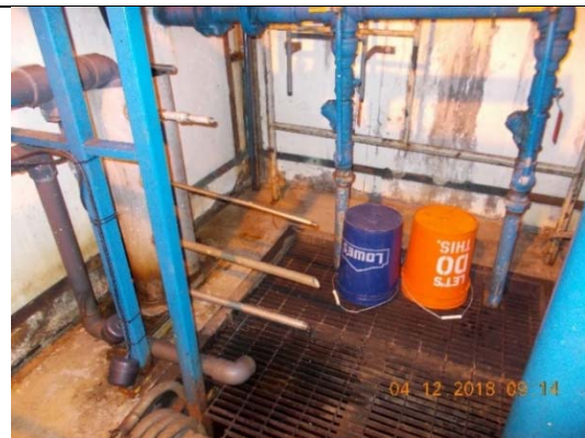
Photo 7: Seal water flow indicators
