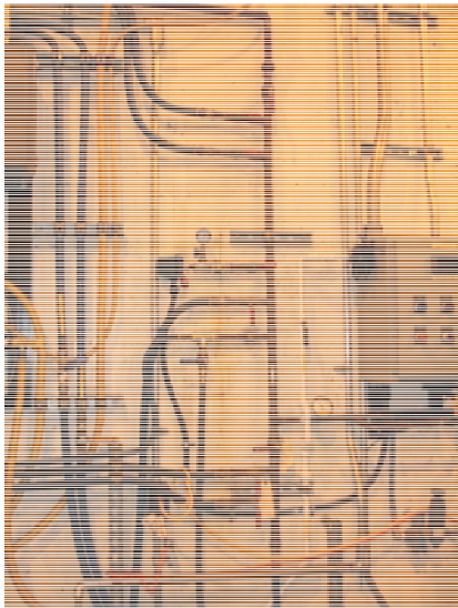
Photo 15: Seal control panel
