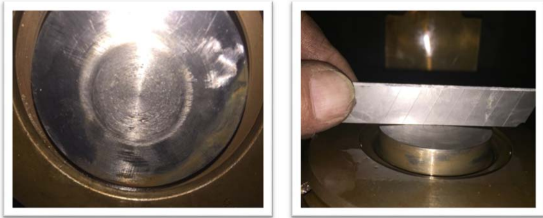
Photos 8 & 9: Damaged load cells. Large amounts of pitting had formed on the top surface.
