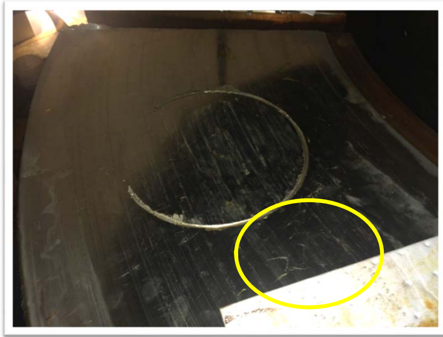
Photo 3: Bearing wiped. Potential cracking on Babbitt pad
