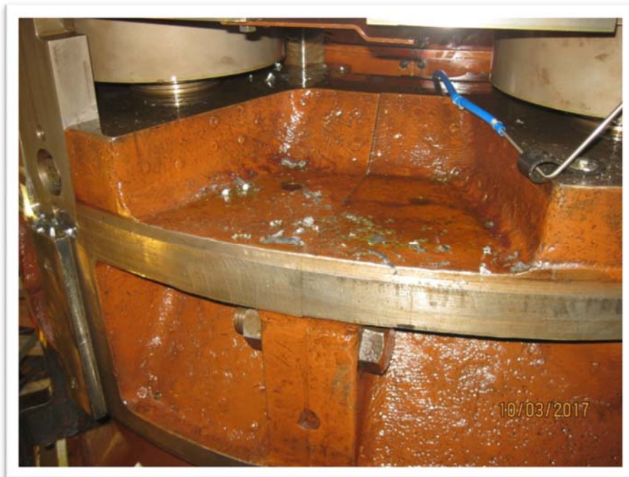
Photo 13: Babbitt chunks located on thrust bearing support base
